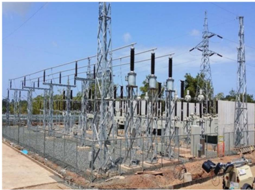
115kV Substation for JINRO Power 57.8MW PPS
