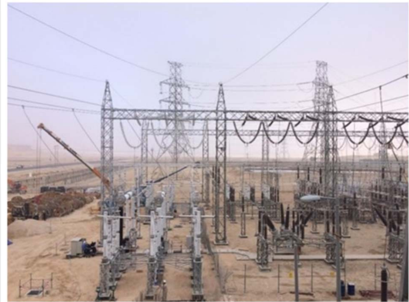
Uthmaniyah Gas Plant (UGP)
