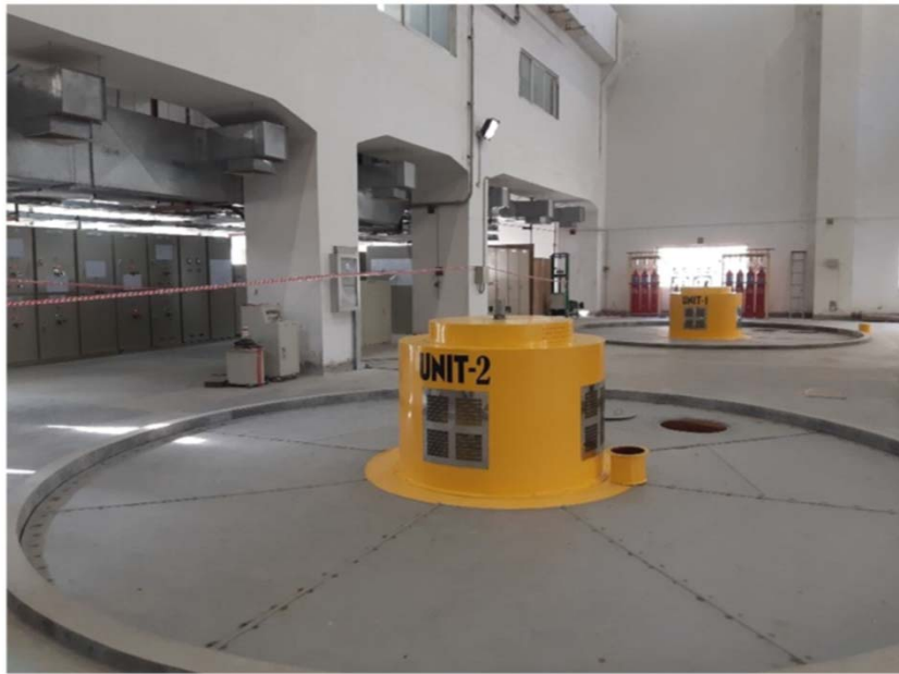
Hydro Power Generator
