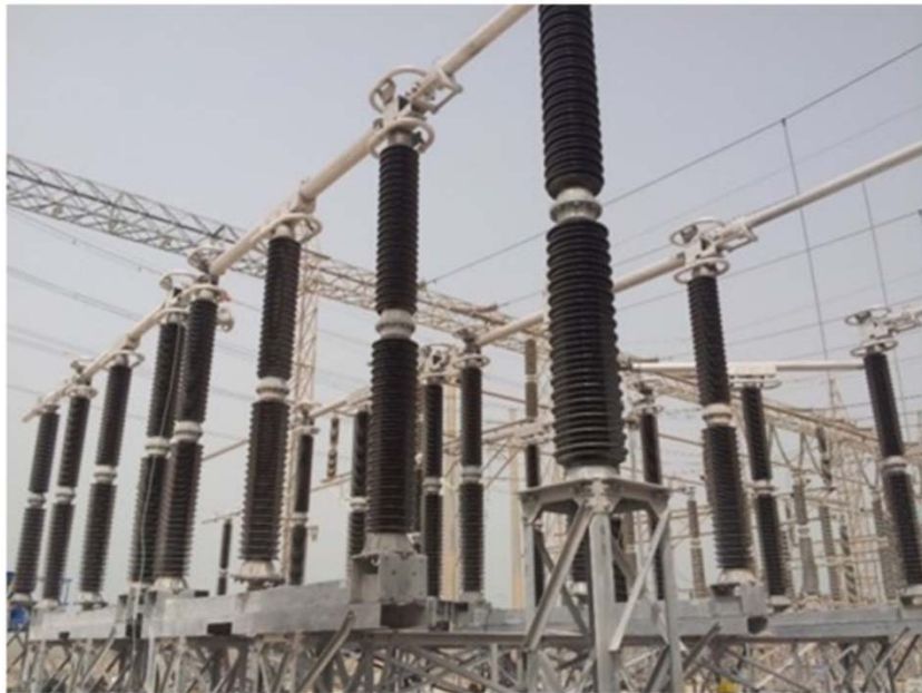
Ju'aymah Gas Plant (JGP)
