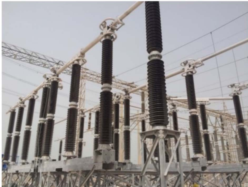
Ju'aymah Gas Plant (JGP)
